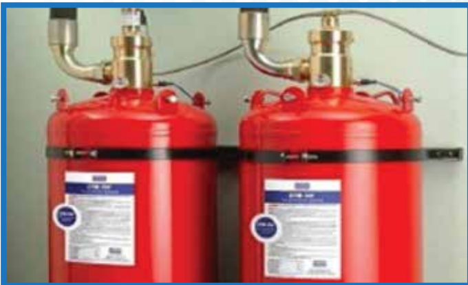
FM200 Piped System
