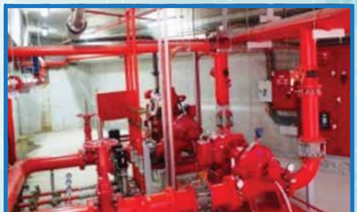
Hydrant/Wet Riser Systems
